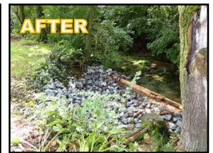
August 2022 – After installation of a modified mudsill. This structure will trap sediment and be covered by vegetation and rebuild the natural stream bank while protecting the bank at the same time.
