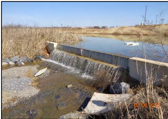
Figure 1: FCCD is facing a challenge when groundwater is encountered during mass earth moving. When a subsurface aquifer is surfaced, developers are challenged with conveying the surplus of water safely to a surface water.
