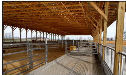
A manure stack pad under construction through CAP funding. This stack pad is attached to a compost bedded pack also under construction.
