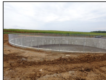
Manure storage tank. This project was funded by the farmer, and our office provide technical assistance for the design and construction oversight.
