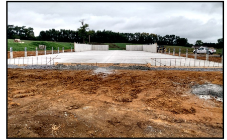
A roofed animal heavy use area with a stack pad under construction through a CEG grant
