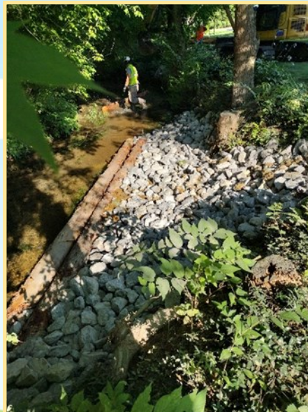
PFBC seasonal technician working to place a log vane after the completion of the modified mudsill in the foreground of the photo.
