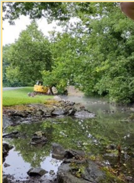
Flyway Excavating, Inc. placing a rock vane in the stream using an excavator. This was the first structure of the project.
