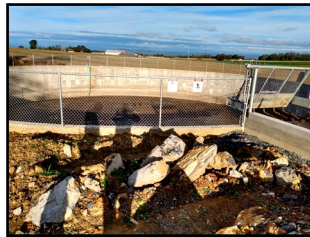
Liquid manure storage tank which replaced an old earthen structure. FCCD provided the survey, design and quality assurance during construction.
