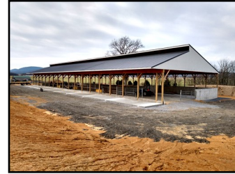
Covered compost bedded pack and stack pad nearing completion. This project was funded through a CAP grant and replaced an old facility that was sending sediment directly to a stream.
