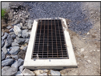
New inlet with filter
