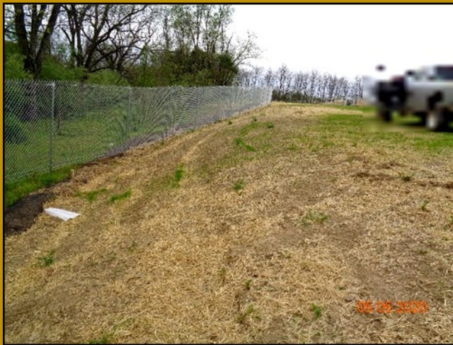
The photo above is a great example of why the District emphasizes the use of erosion control matting on steep slopes. As you can see, there was no matting used, vegetation is sparse, and the compost filter sock is overwhelmed with accumulated sediment.
